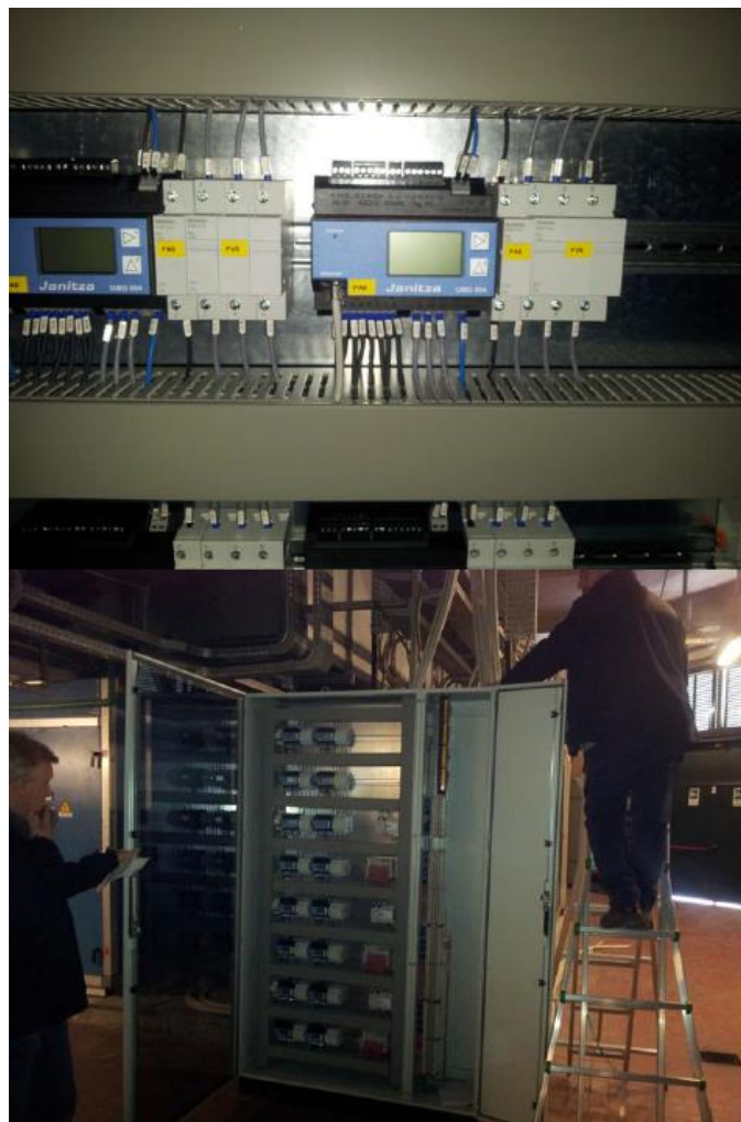
Figure 4: Data acquisition system at Fiumicino airport. Advanced Data Logging Systems for the measurement of energy flows, temperature, pressure and humidity have been developed by CASCADE and installed at the airport pilots.
